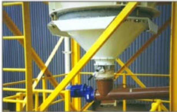
Bin Activator, Silo Discharge
